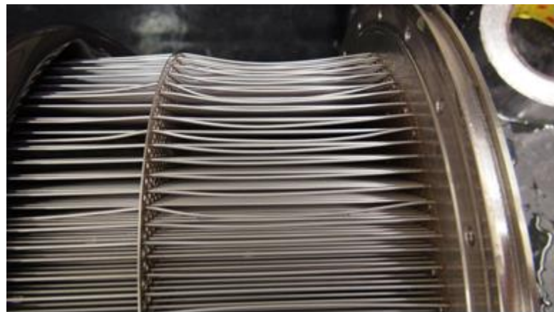
Figure 10. Tube deformation due to thawing.
