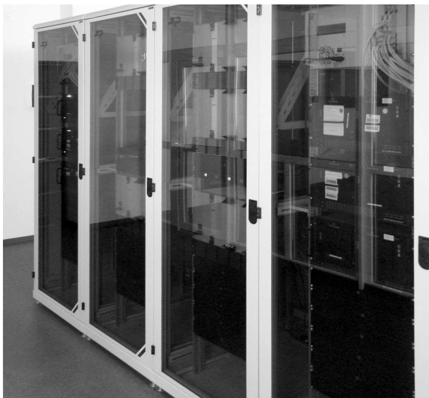
Figure 1. View of the six-station ARC correlator, showing four racks containing (left to right) signal distribution and synchronization system (SDSS) and three Mark 5B playback units, two correlator crates and KVM, three correlator crates, and one more cabinet with SDSS and three Mark 5B playback units.
