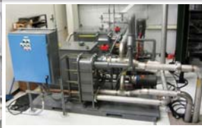
Cooling Water System provides 2 separate systems that cool induction coil and power feedthrough, induction heater and H 2 N 2 mixer respectively
