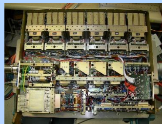
Efficient, high voltage power processors
