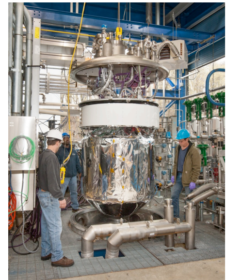
Liquid Hydrogen (LH 2 ) RBO Experiment Test Article Being Lowered into SMiRF Vacuum Chamber. The white ring above the test tank is the heat pipe radiator, behind which is mounted the reverse turbo-Brayton cycle cryocooler.
