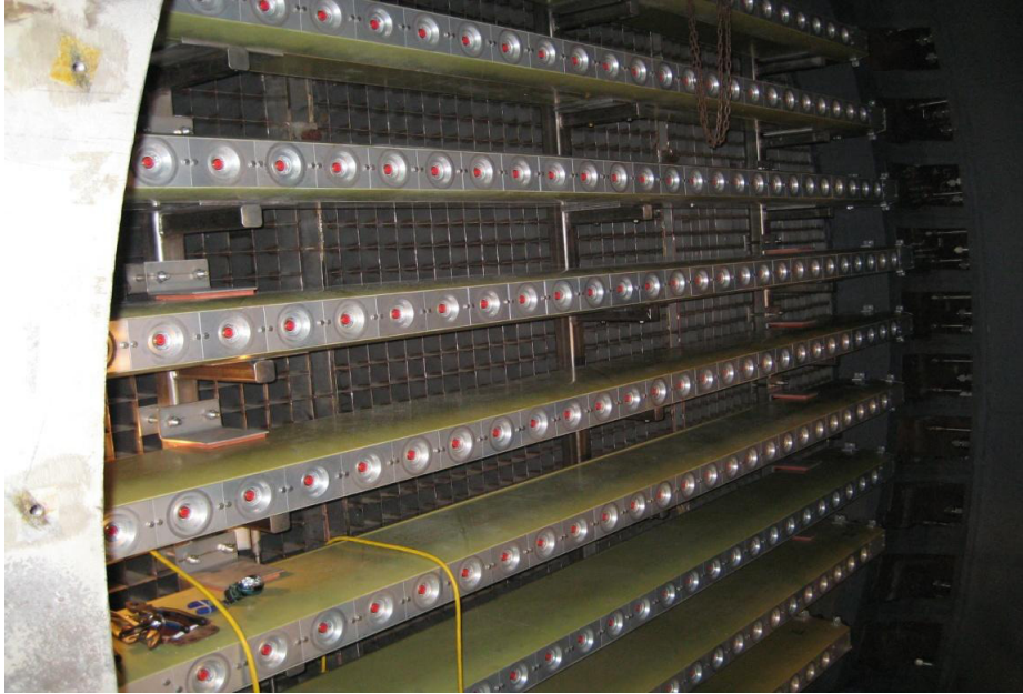
Spray Bars Installed in Plenum
