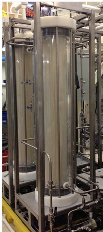
Figure 1. Assembled and installed MABR
