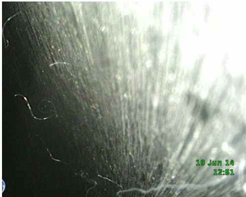
AR Borescope Photos
