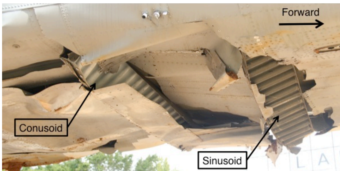
Figure 32. Post-test photograph of the outer belly skin deformation between FS220 and FS286.
