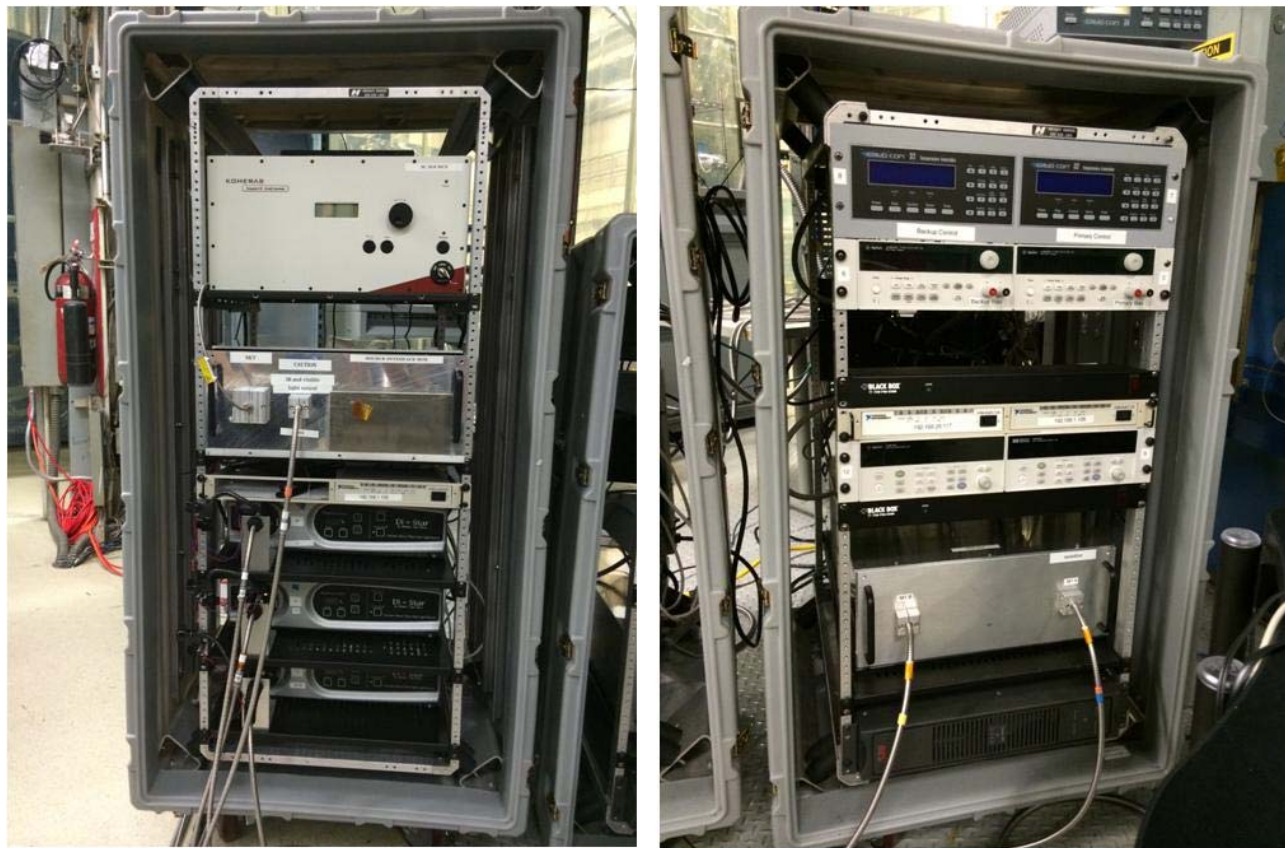
Figure 2. JPSS FPI racks with sources, control electronics, and communications. Rack 1 is on the left; Rack 2 on the right.
