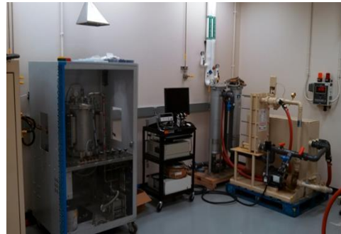
Figure 4. Compact Fuel Element Environmental Test facility (CFEET)
