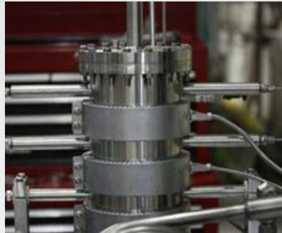
RWGS Reactor (prior to installation of insulation)
