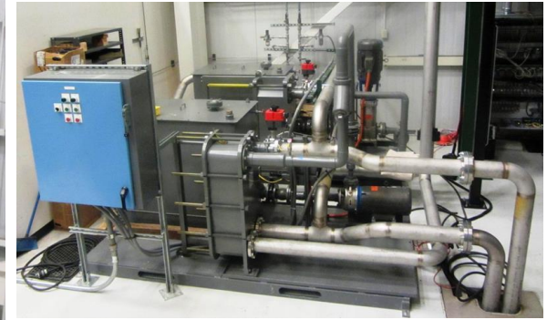
New Cooling Water System now provides 2 separate systems that cool induction coil and power feedthrough, induction heater and H 2 N 2 mixer respectively
