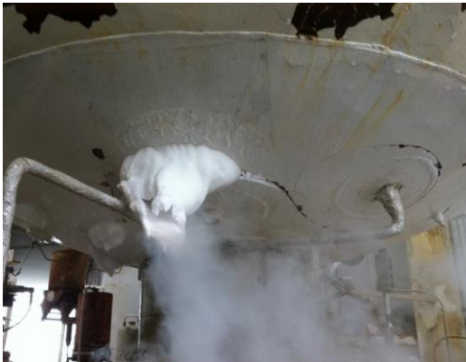
Figure 3. Picture of B-1 tank cracks
