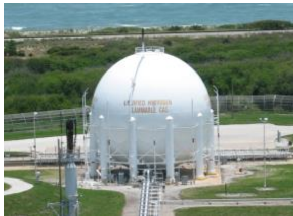
Figure 2. LC-39 Pad A LH 2 Storage Tank
