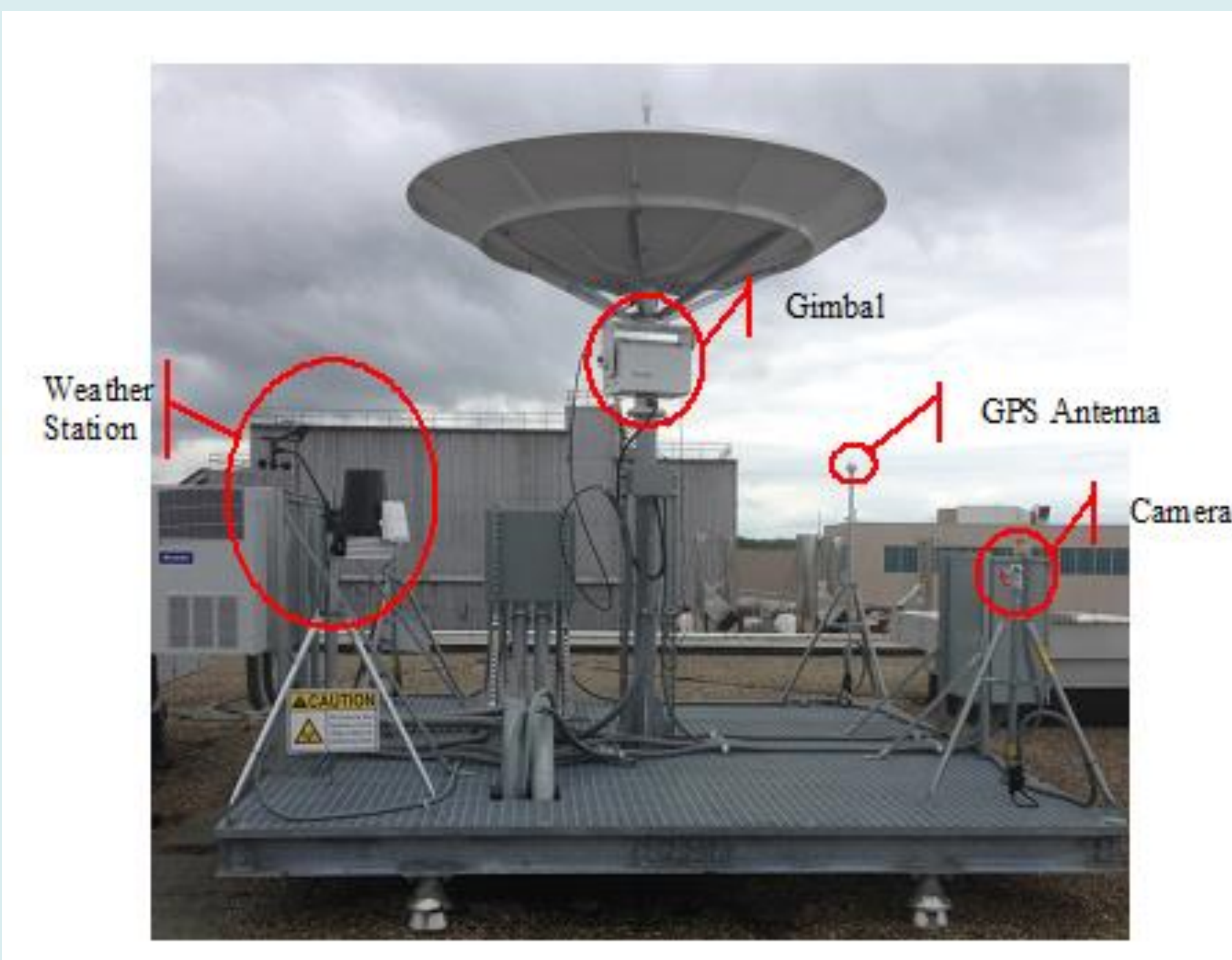
GRC-GS Equipment Located on the Roof of Building 110 at the Glenn Research Center
