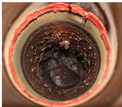
Figure 5. Middle of UBDS system (above baffles).
