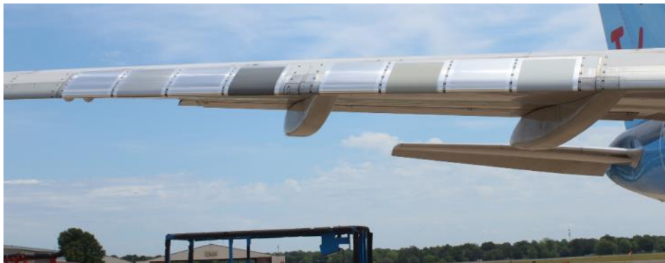
Figure 38: Complete IAM Panel Installation
