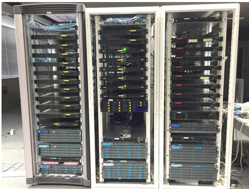
Fig. 2 View of the existing data processing servers.
