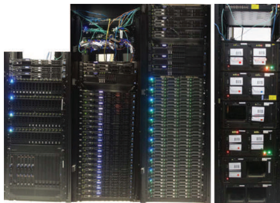
Fig. 2 DiFX cluster system and Mark 5A/B units.
