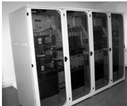
Fig. 1 View of the six-station ARC correlator, showing four racks containing (left to right) signal distribution and synchronization system (SDSS) and three Mark 5B playback units, two correlator crates and a KVM, three correlator crates, and one more cabinet with an SDSS and three Mark 5B playback units.
