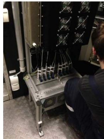
Fig. 6 The BRAS on the RT-13 radio telescope at the Badary observatory.
