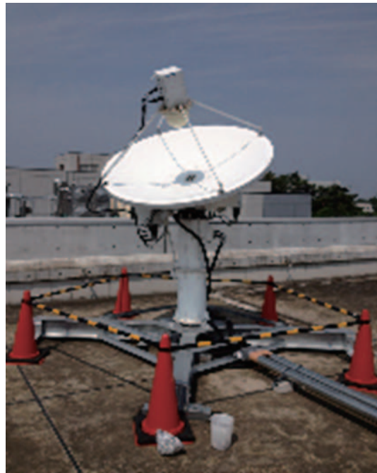
Fig. 1 The MARBLE1 compact station on the roof of the NMIJ building in Tsukuba.
