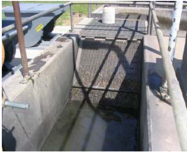
Figure 5. View of the Grit Removal Chamber
