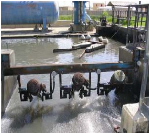
Figure 6. View of the Skimmer and Mechanical Mixers
