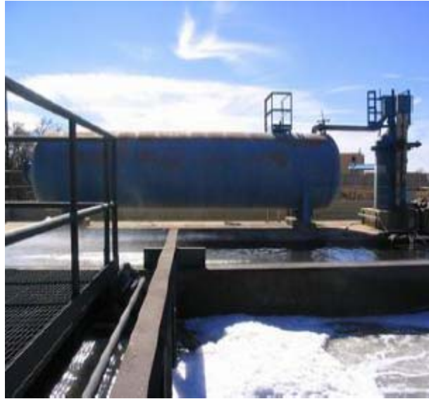
Figure 7. View of Oil -Water Separator
