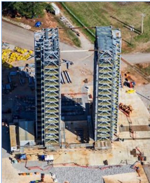
Figure 5. Top, LOX Test Stand 4697 under construction. Bottom. Outfitting under way on LH2 Test Stand 4693, early 2016.
