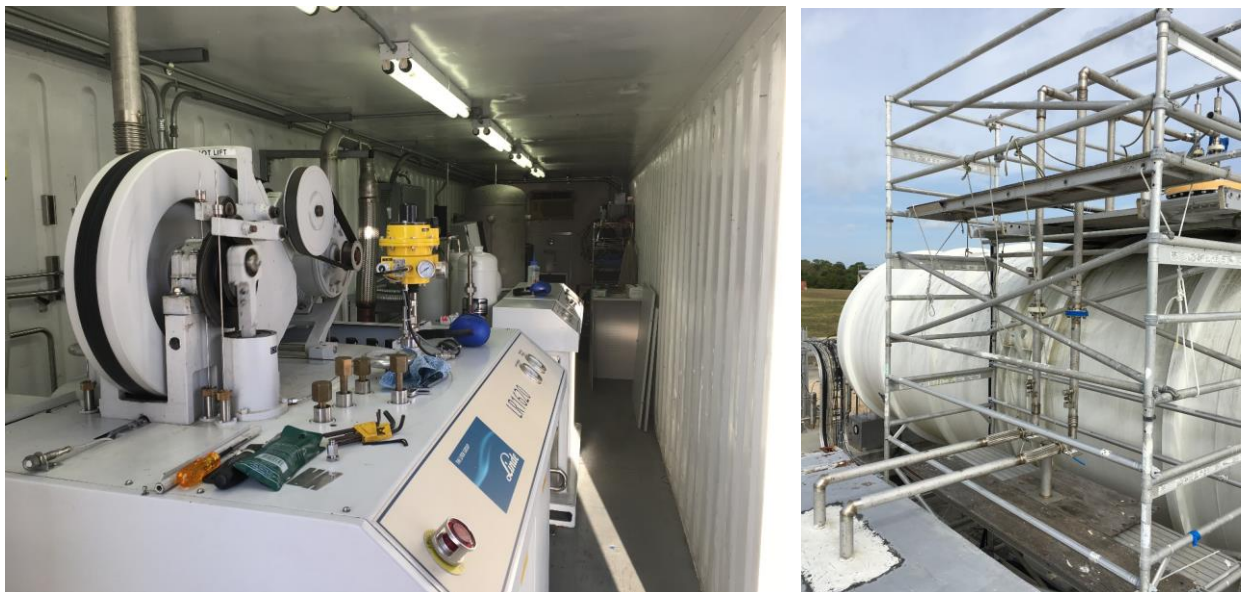
Figure 4: Refrigeration Container Showing the Refrigerator Module (foreground) and RSX Compressor (background) (left); GHe VJ Piping Interfaced to IRAS Tank (right)
