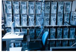
FIGURE 5.2: Networking and Power for Eridani: Hot Isle
