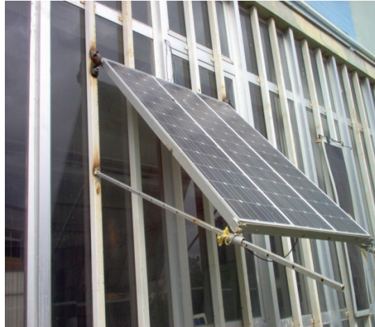
FIGURE 5. Three PV modules hinged on a window with an adjustment of inclination
