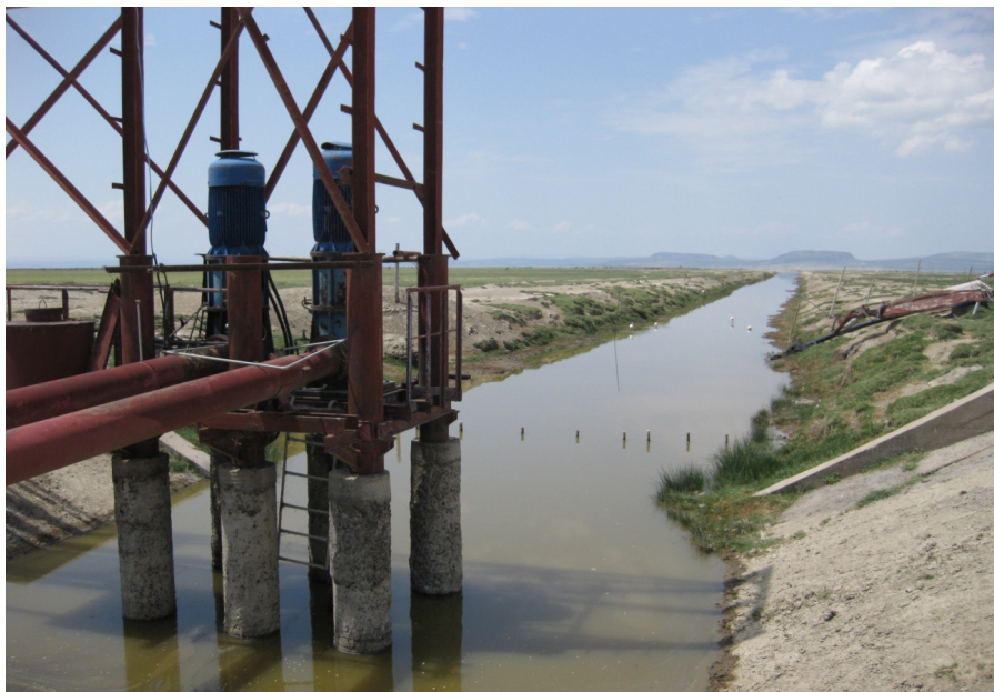
Figure 41. Pumping station of the soda ash factory. Author: Ester Raventós
