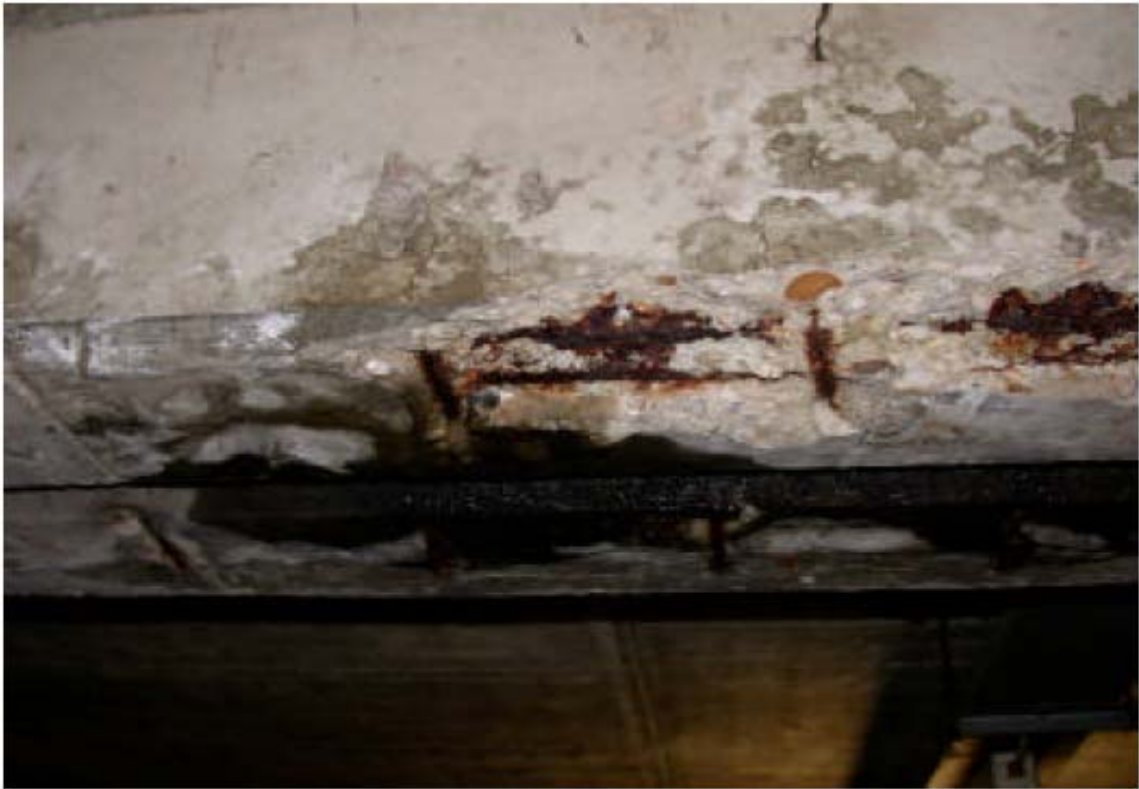
Figure 2.10 reinforcement corrosion caused by chloride ingress [21]
