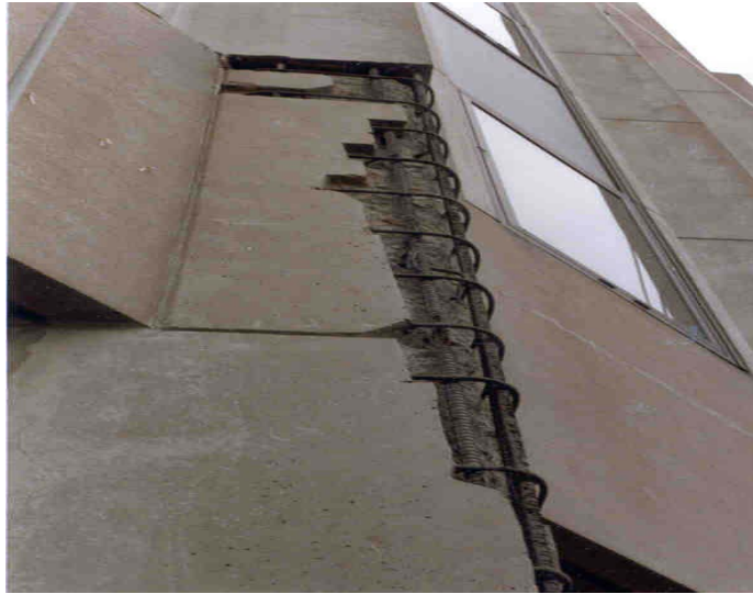
Figure 4.10 Removal of defected concrete for replacement Genesee Hospital Doctor's Building - Rochester, New York [29]
