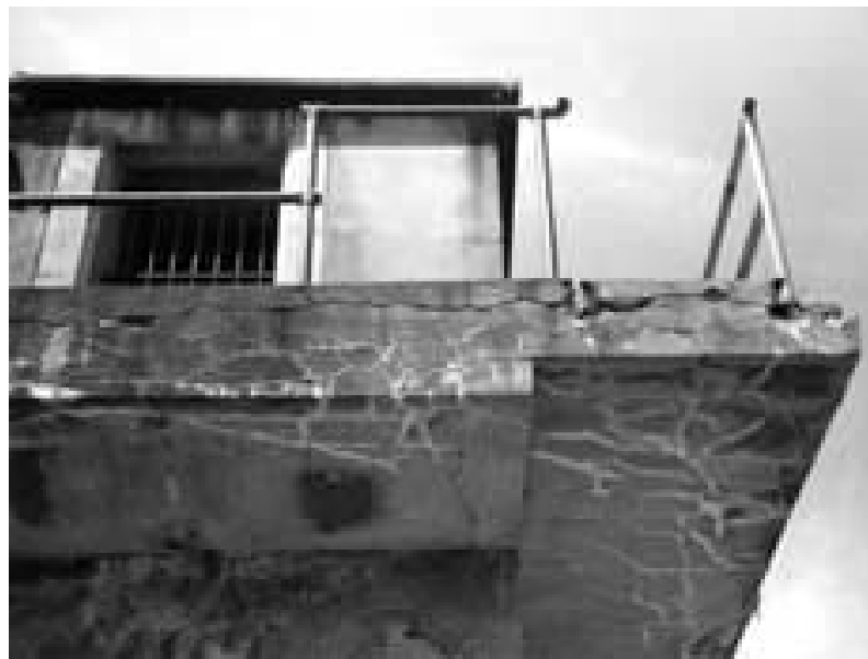
Figure 2.36 the 1904 reinforced concrete tower deteriorated due to freeze thaw and reinforcing steel corrosion [33]
