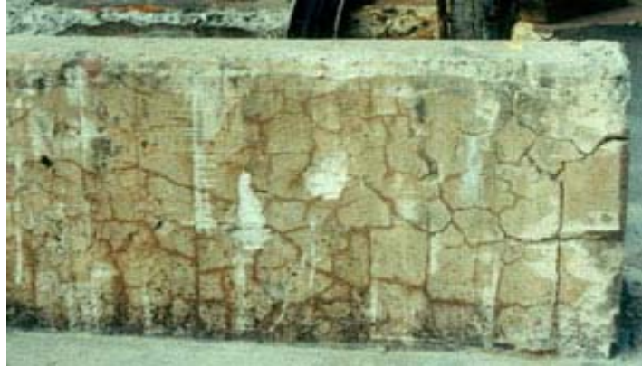
Figure 2.33 ASR-Induced Damage in Unrestrained Concrete Element. Uniform Expansion in all Directions Results in Classic Map-Cracking [26]
