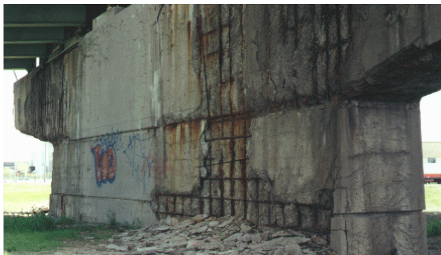
Figure 2.18 Corrosion damage in a North American elevated highway structure exposed to de-icing salts - notice spalling of the concrete cover, leaving the rebar exposed [38]
