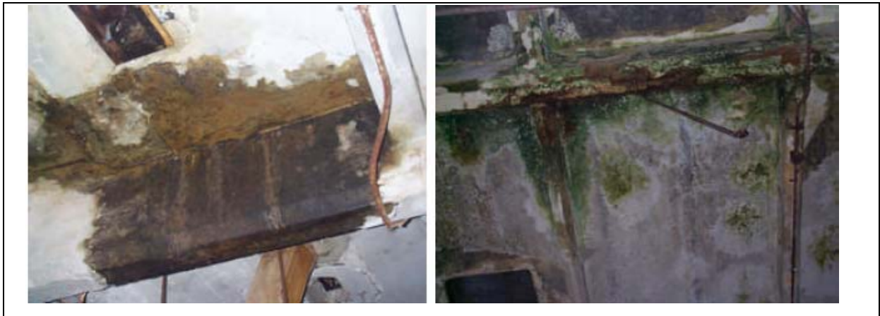
Figure 8.6 Damaged concrete (left) and moss growth on the structure (right)
