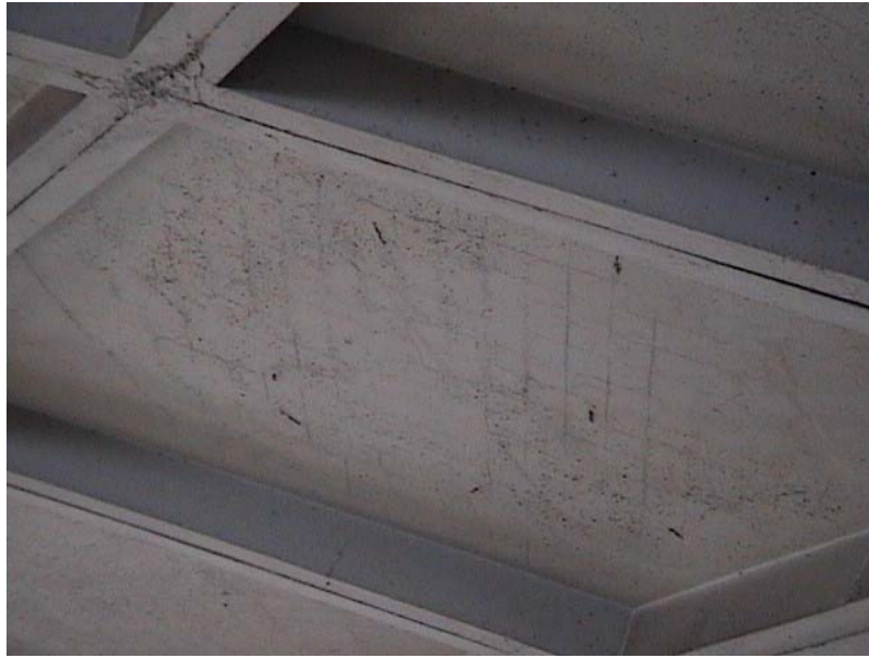
Figure 8.20 grid cracks of the under side of the thin reinforced concrete shell elements
