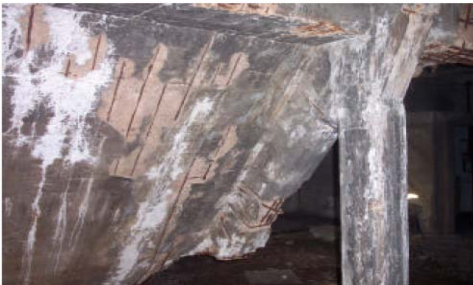
Figure 2.16 reinforcement corrosion caused by carbonation of concrete [21]
