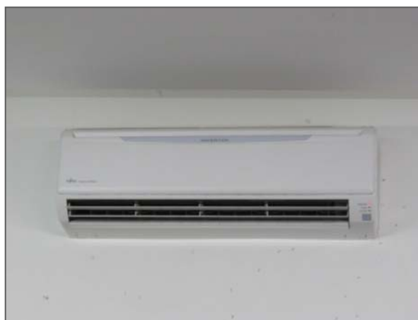
FIGURE 8-76. THE HEAT PUMP IN THE ROSENEATH CLASSROOM.
