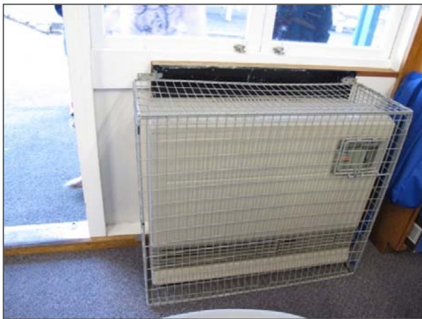
FIGURE 8-75. THE GAS-HEATING UNIT IN THE NORTHLAND CLASSROOM.
