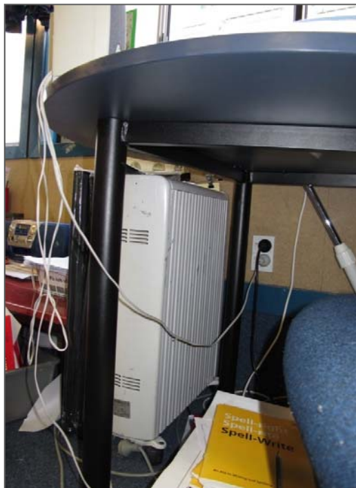
FIGURE 8-73. THE ELECTRIC HEATING UNIT IN THE CLYDE QUAY CLASSROOM.
