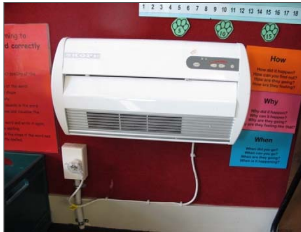
FIGURE 8-74. THE SMALL ELECTRIC HEATING UNIT IN THE THORNDON CLASSROOM.
