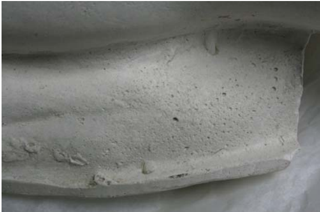
Fig. 1 Detail of a plaster surface characterized by a widespread porosity.
