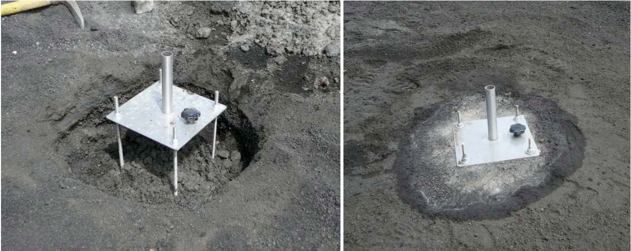
Figure 5. CR base positioning on the ground. Left figure highlights the four rods drowned in the cement, right figure shows the final positioning of the base.
