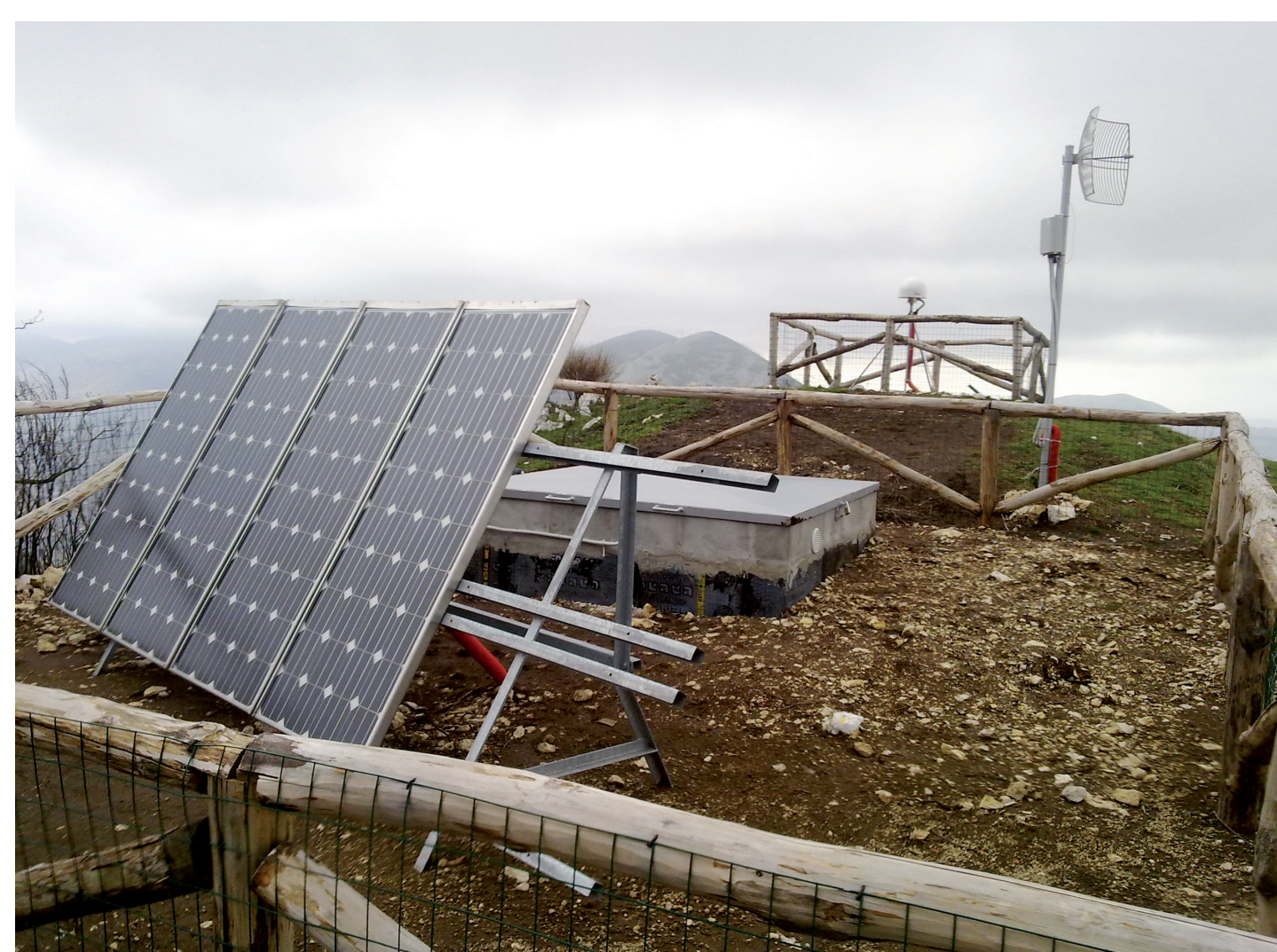
Fig. 1 - Example of a remote station.
