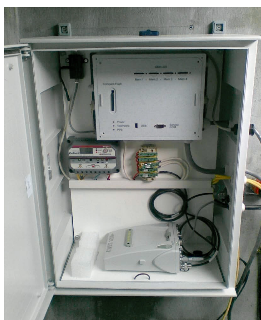
Fig. 2 - Example of a remote cabled site.
