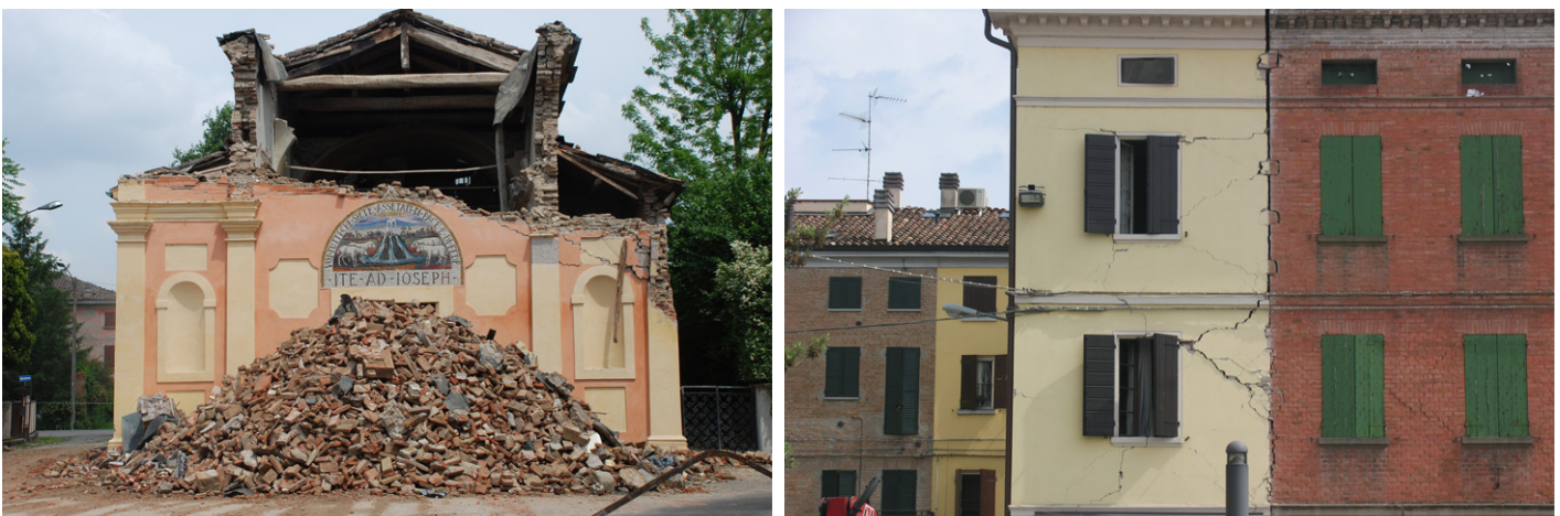
Figure 3. a. Partial collapse of a monumental building: the S. Giuseppe church in San Felice sul Panaro. b. Widespread cracks in a class B building in Cavezzo.
