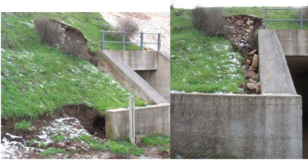
Fig. 17. Photos of the concentrated erosion pipe at the contact between the wall of the concrete conduit and the soil material.
