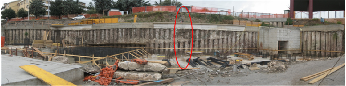
Figure 1. The Student House in Campobasso, Vazzieri - University of Molise. The monitored flexible retaining wall and sensor location (Rainieri et al., 2010).
