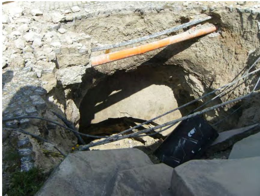
Figure 60. In the foreground of Figure 59 at the top of the hill in the center of Castelnuovo, a large sinkhole formed beneath the road exposing the weakly cemented Pleistocene sandstone that underlies the village. Water draining through the sinkhole was actively eroding a large void approximately 3-5 m in diameter and at least 6 m in depth. Cementation was strong enough to support small overhangs, at least temporarily (42.2947°, 13.629°).
