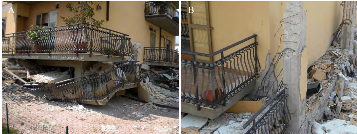
Figure 74. San Gregorio eastern part. (A) RC building “pancake” collapse, (B) Detail of sheared pillars.
