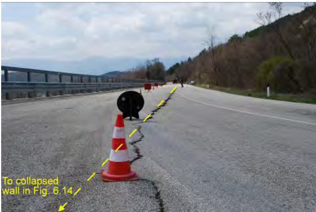
Figure 190. Pavement cracking in SS80 roadway (from L' Aquila to Campotosto) in the location of collapsed masonry retaining wall ( 42.420510^{\circ}\text{N} , 13.358394^{\circ}\text{E} ).
