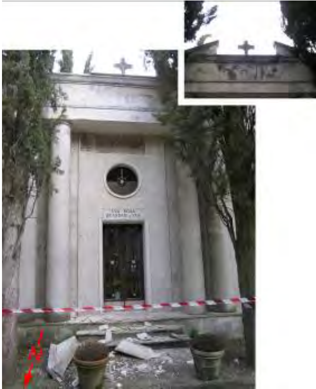
Figure 52. Breakage and fall of ornamental objects from a tomb roof.
