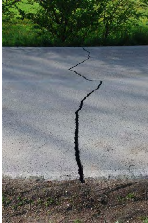
Figure 142. Typical tensile condition of road cracks, not extending into neighboring sub-base or approach fill embankment (42.324N, 13.478E).
