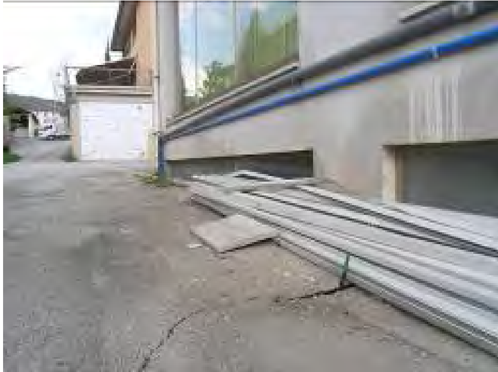
Figure 32. Ground fissures and settlement at the side of the building (42.359817°N, 13.468649°E).
