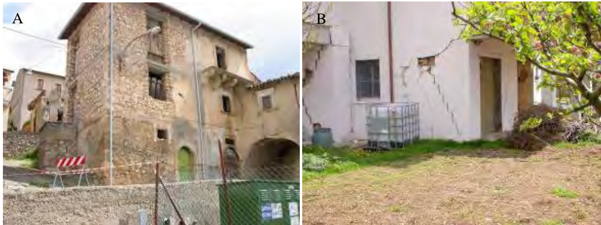
Figure 96. Barisciano. (A) Collapse (D5) of an old masonry building in background, (B) Damages (D1/D2) to RC buildings.
