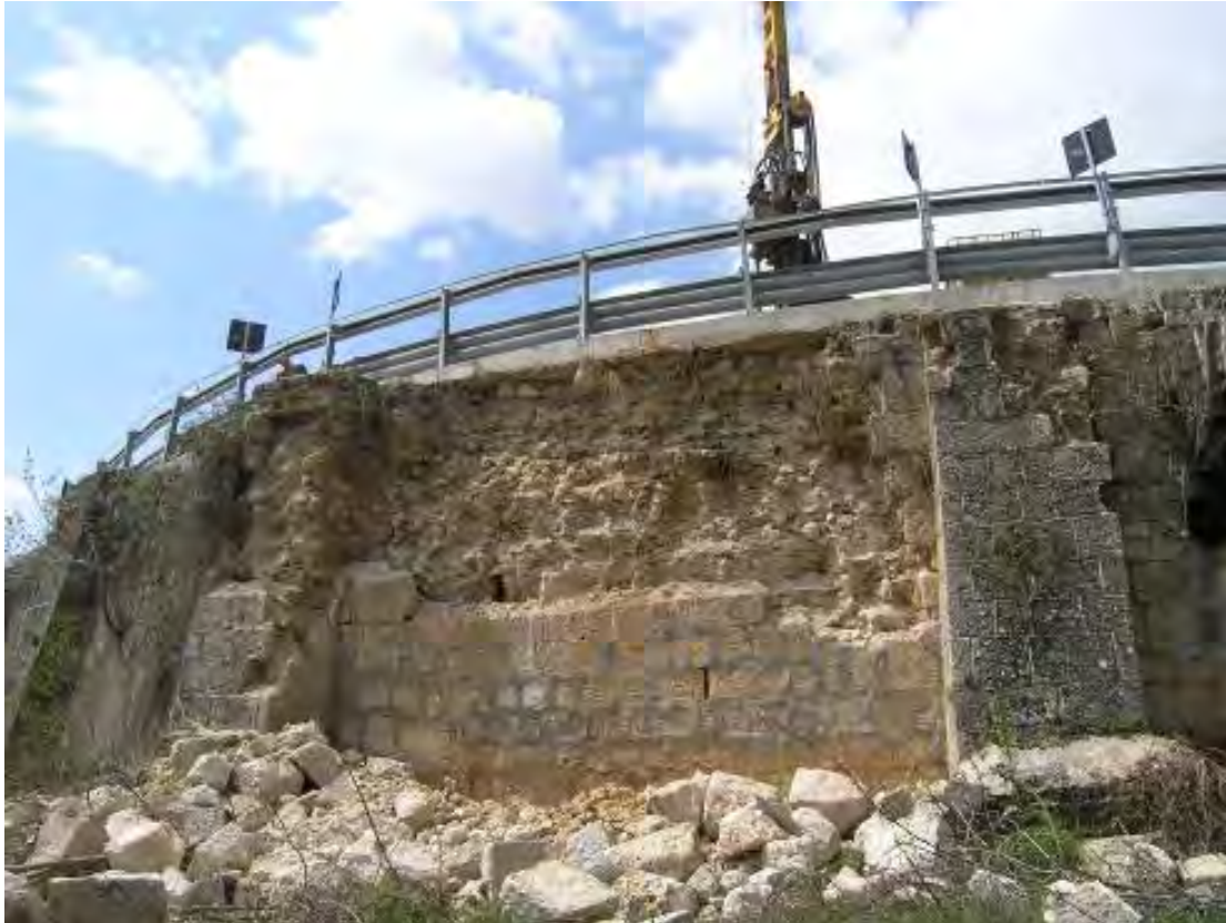
Figure 189. Partially collapsed wall at SS80 highway between L'Aquila and Campotosto ( 42.420510^{\circ}\text{N} , 13.358394^{\circ}\text{E} ).
