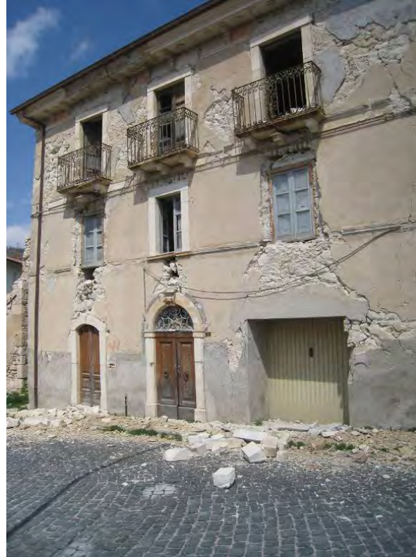
Figure 58. A typical heavily damaged structure in the lower elevation of Castelnuovo. Many structures in the lower elevation neighborhood had less observable damage. (42.2956°, 13.6274°).
