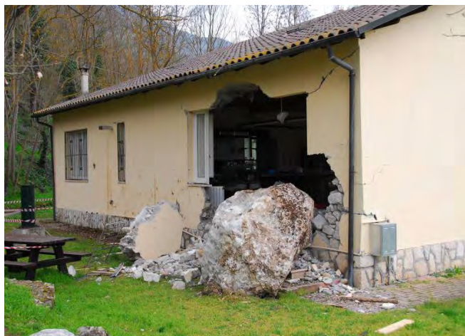
Figure 114. Rock fall impact at the Caves of Stiffe (42.255N 13.547E).
