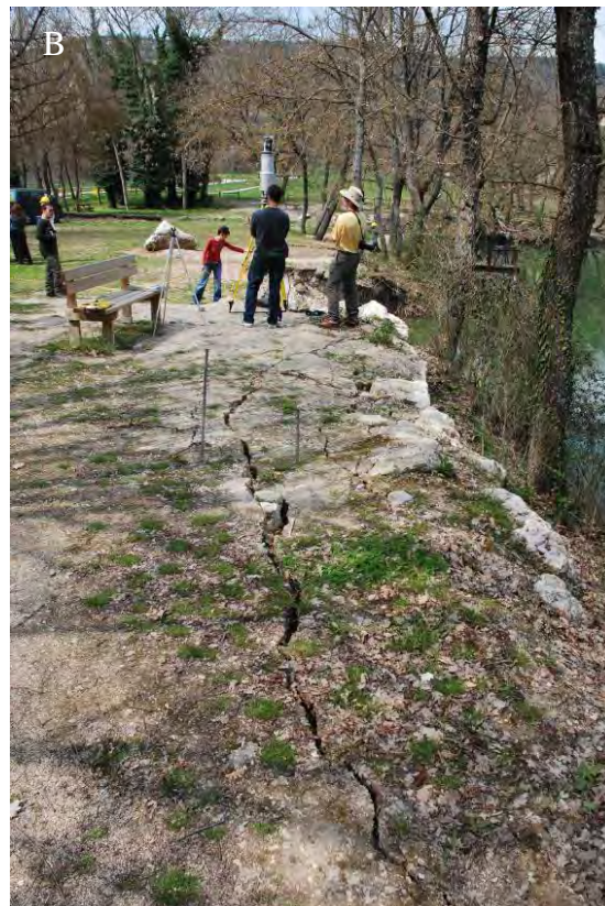
Figure 162. Ground cracks at the southwest corner of Lake Sinizzo (location WP 18) as observed on (B) 15 April 2009.
