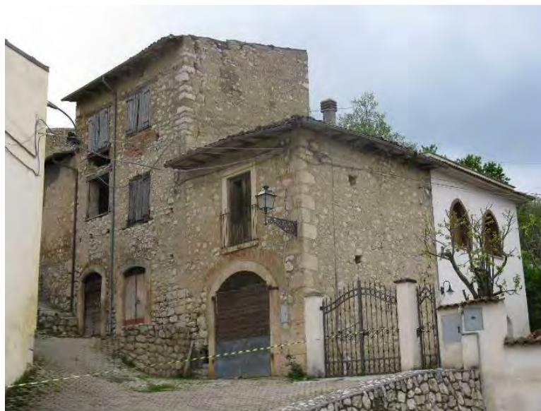
Figure 83. Casentino masonry buildings with some wall cracks.
