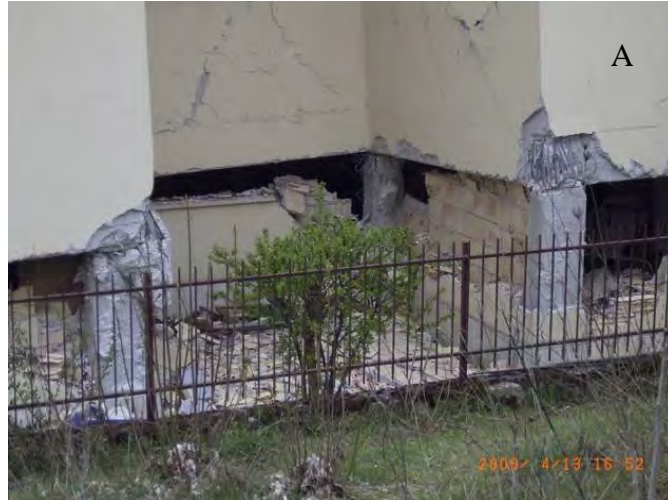
Figure 110. Damage on the structures in the cluster in zone (d). (A) Waypoint GB-24-1 (D5).
