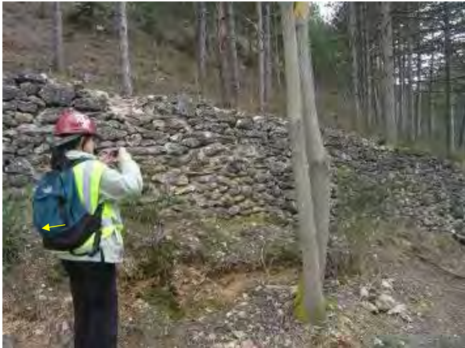
Figure 185. Minor damage on masonry wall in severely shaken Pettino area ( 42.374011^{\circ}\text{N} , 13.367498^{\circ}\text{E} ).
