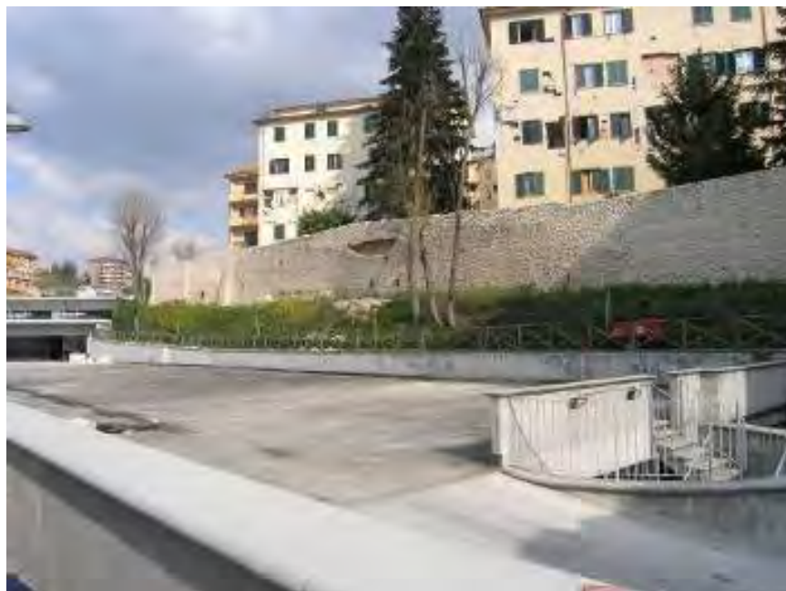
Figure 188. Damaged wall at downtown L'Aquila ( 42.356056^{\circ}\text{N} , 13.389524^{\circ}\text{E} ).
