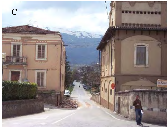
Figure 70. Monticchio. (C) D1 damage (fall of the cornice) on a masonry building.
