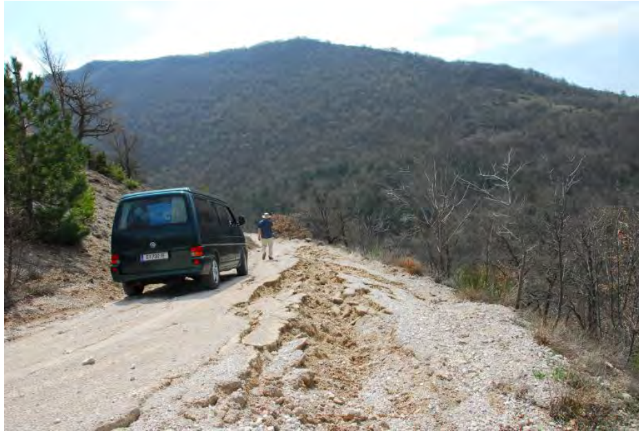
Figure 138. Failure of side-hill fill embankment (42.420N 13.376E).
