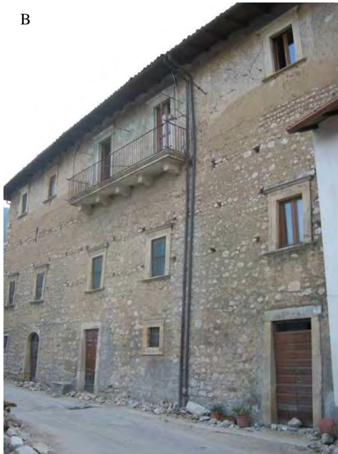
Figure 88. Villa S. Angel. (B) Reinforced masonry in the historic center with minor cracks in the highest story (D2).
