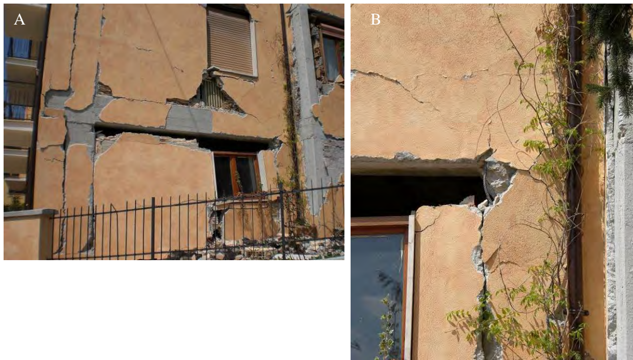
Figure 75. San Gregorio eastern part. (A) RC building with structural damage, (B) Detail of the damage to the beam-column connection.
