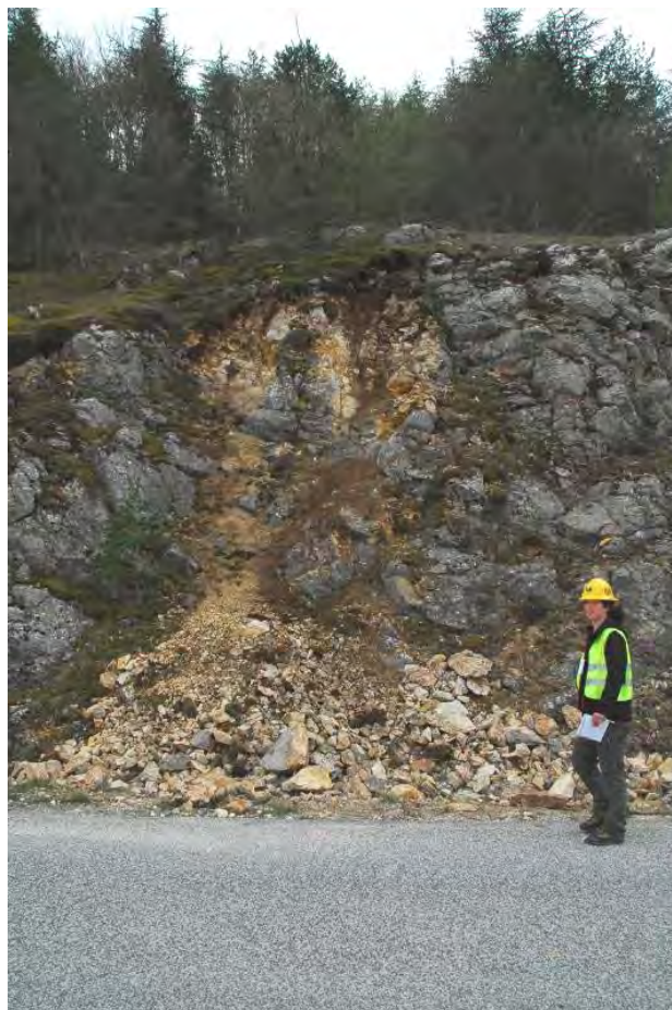
Figure 118. Shallow ravelling-type failure of weathered limestone blocks (42.278N, 13.468E).
