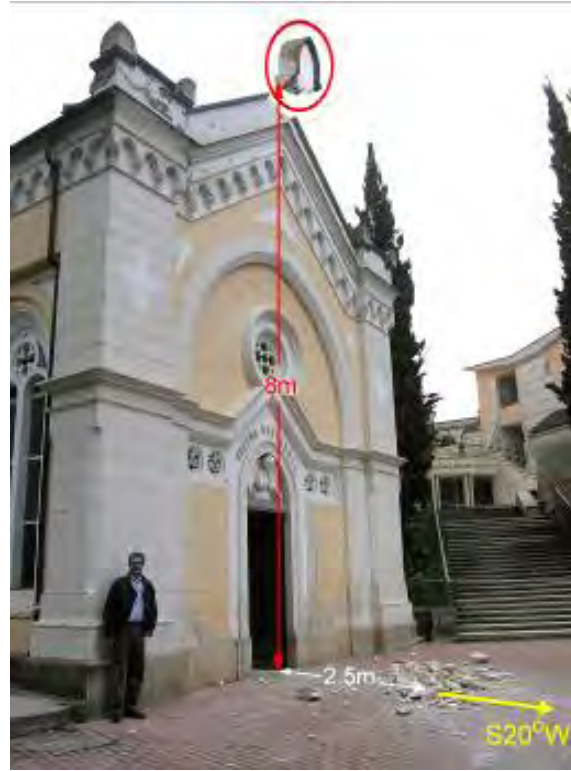
Figure 53. Fall of facade object at mortuary building.
