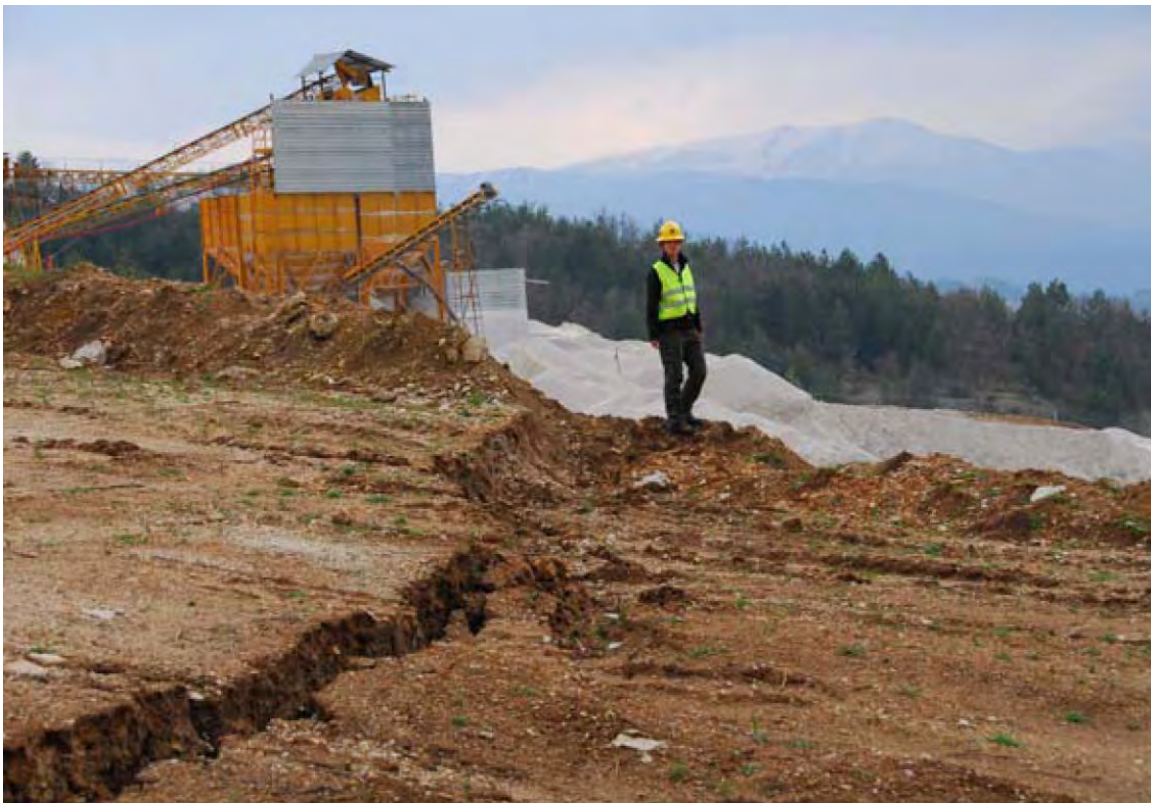
Figure 149. Shear failure developed in fill material, with vertical displacement increasing to approximately 40 cm at free slope face (42.435N, 13.330E).
