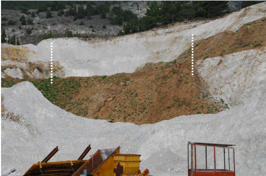
Figure 151. Graben structure (between vertical lines) and bedrock boundary conditions (42.435N, 13.330E).
