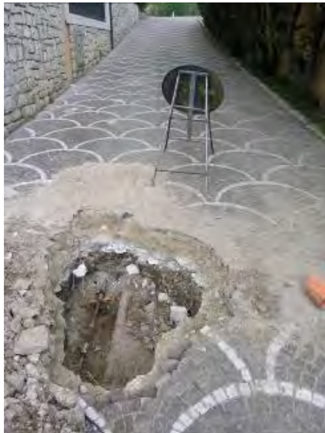
Figure 29. Failure of water pipe. (42.359335°N, 13.468954°E).
