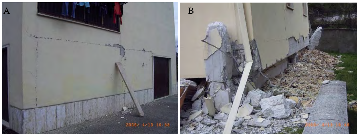
Figure 109. Damage on the structures in the cluster in zone (d). (A) Waypoint GB-22-1 (D1), (B) Waypoint GB-23-1 (D5).
