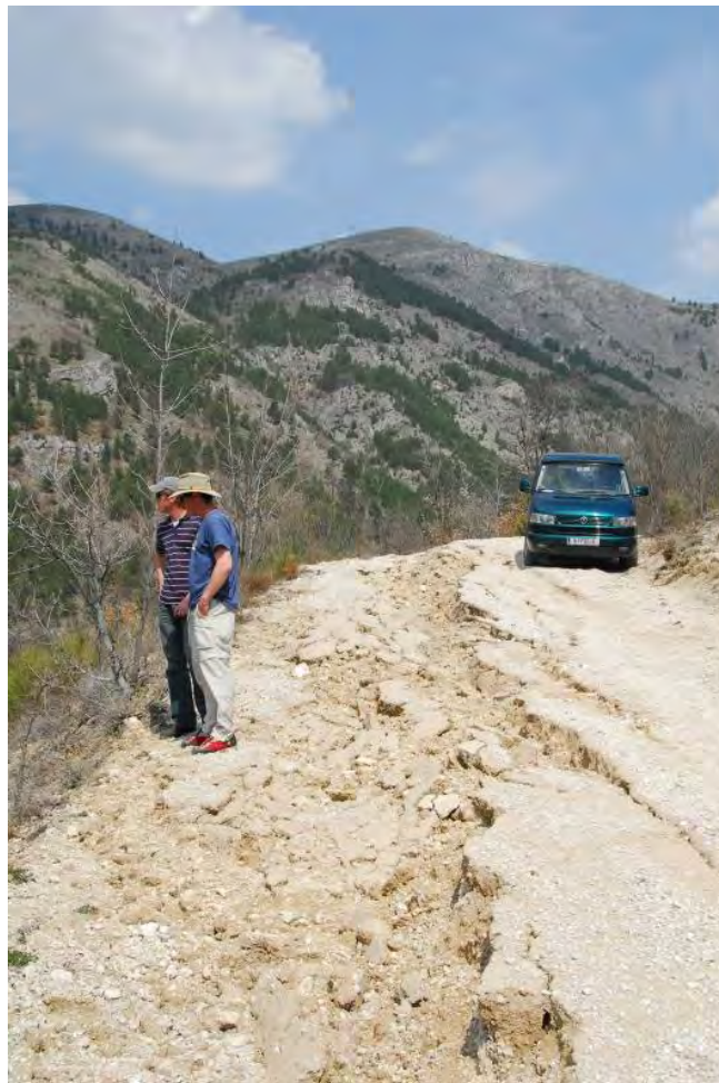
Figure 139. Failure of side-hill fill embankment (42.420N 13.376E).
