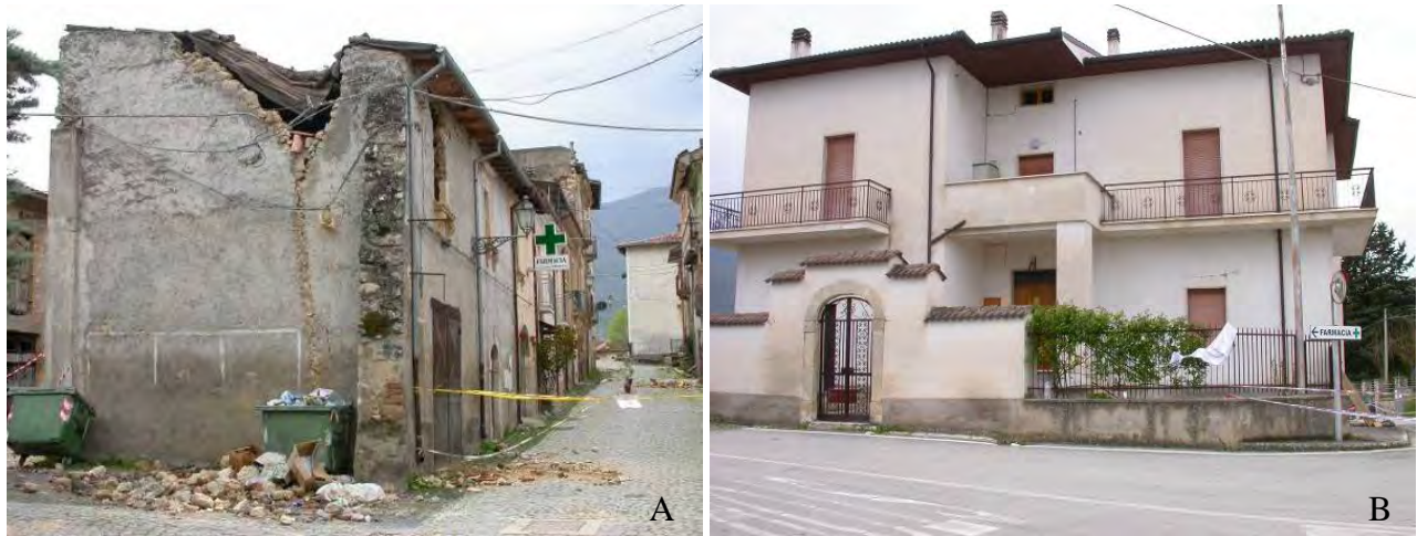
Figure 79. S. Eusanio Forconese village. (A) Partial collapse of masonry building (D4), (B) Slight damage to a RC building nearby (D1).
