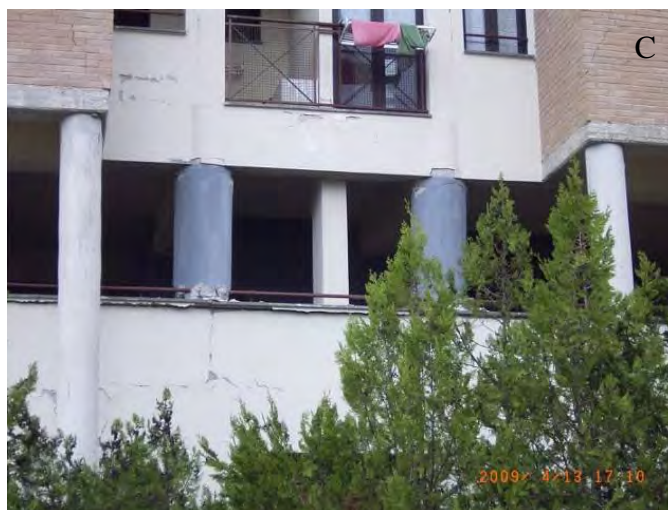
Figure 110. Damage on the structures in the cluster in zone (d). (C) Waypoint GB-26-1 (D2).
