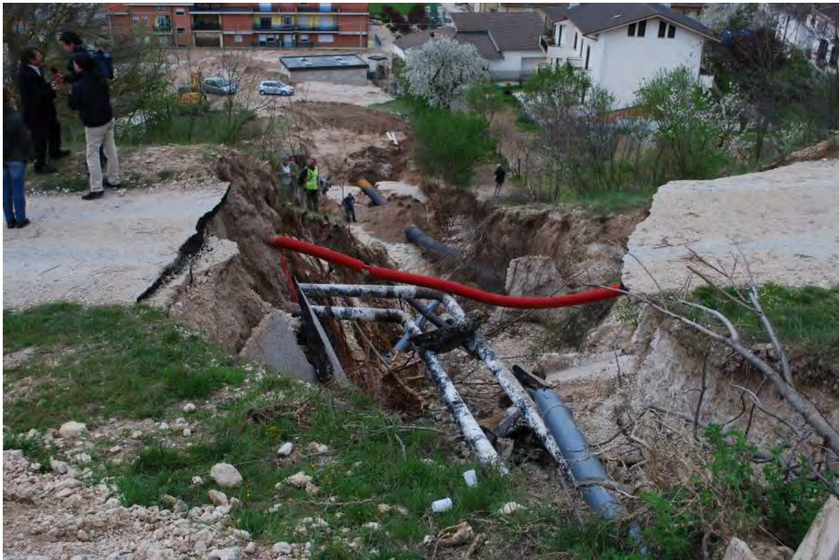
Figure 27. Paganica village: broken major water pipe (repaired) due to co-seismic rupture (Lat. 42,36537N Long. 13,46803E) (Photo by Mylonakis G).
