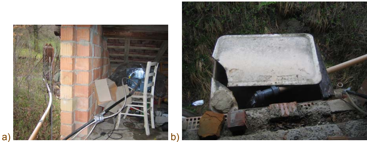
Fig. 3 a): The Miano station with the gas/water separator on the left site, the tube to the house and the drum gas counter on the right site. 3b): The water outlet at the house with the water temperature probe and the water flow sensor.
