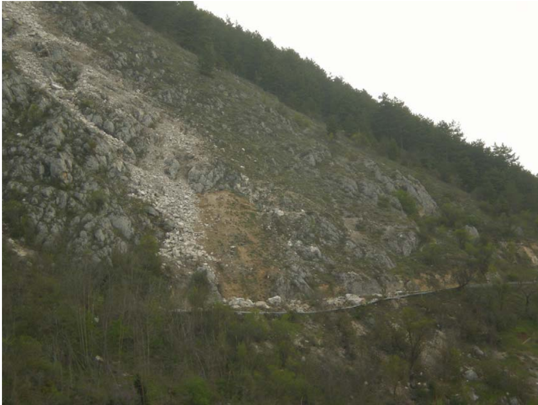
Figura 42 Pareti di distacco e grossi massi calcarei crollati (WPT RN10 42.3171/13.4705). Figure 42 Surface of detachment and mass fall (WPT RN10 42.3171/13.4705).
