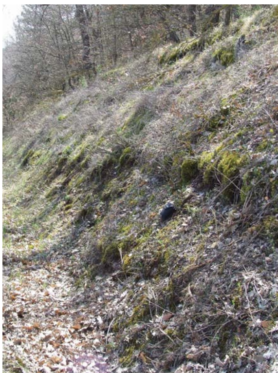
Figure 31 Fissuring and soil detachment from the bedrock fault plane (WPT SP36, 42.3051/13.4105).
