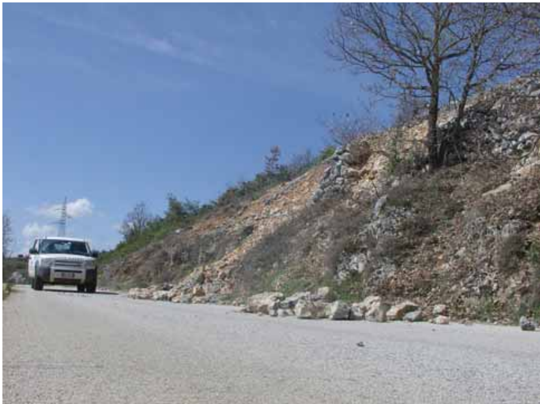
San Giacomo, crolli a bordo strada San Giacomo, rock fall by the roadside
