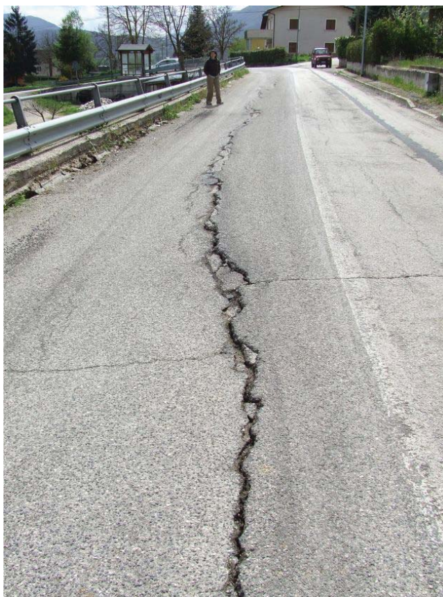
Figura 47 Frattura lungo la strada Casentino-Tussillo (WPT RN15, 13.5312/42.2692). Figure 47 Break in the paved road Casentino-Tussillo (WPT RN15, 13.5312/42.2692).
