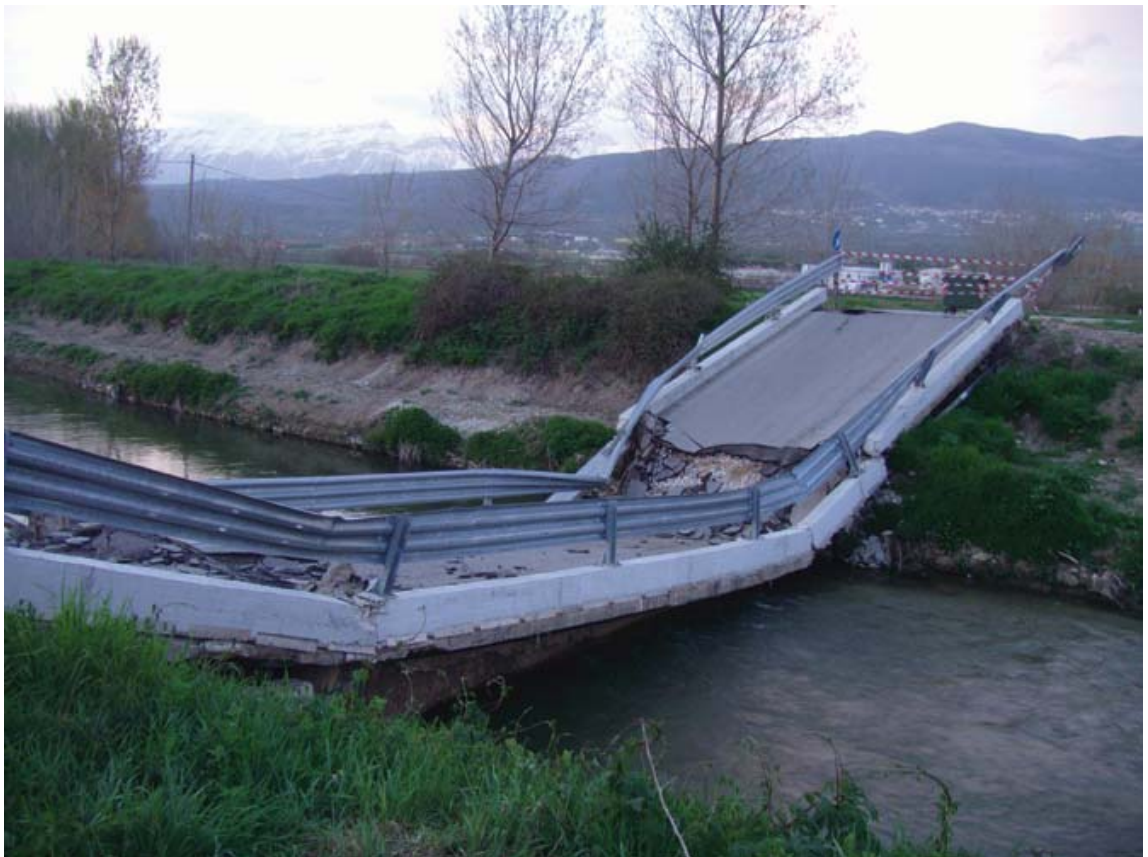
Figura 55 Ponte crollato sul Fiume Aterno, WPT CB63, 42.3039/13.5029). Figure 55 Collapsed bridge over the river Aterno, WPT CB63, 42.3039/13.5029).
