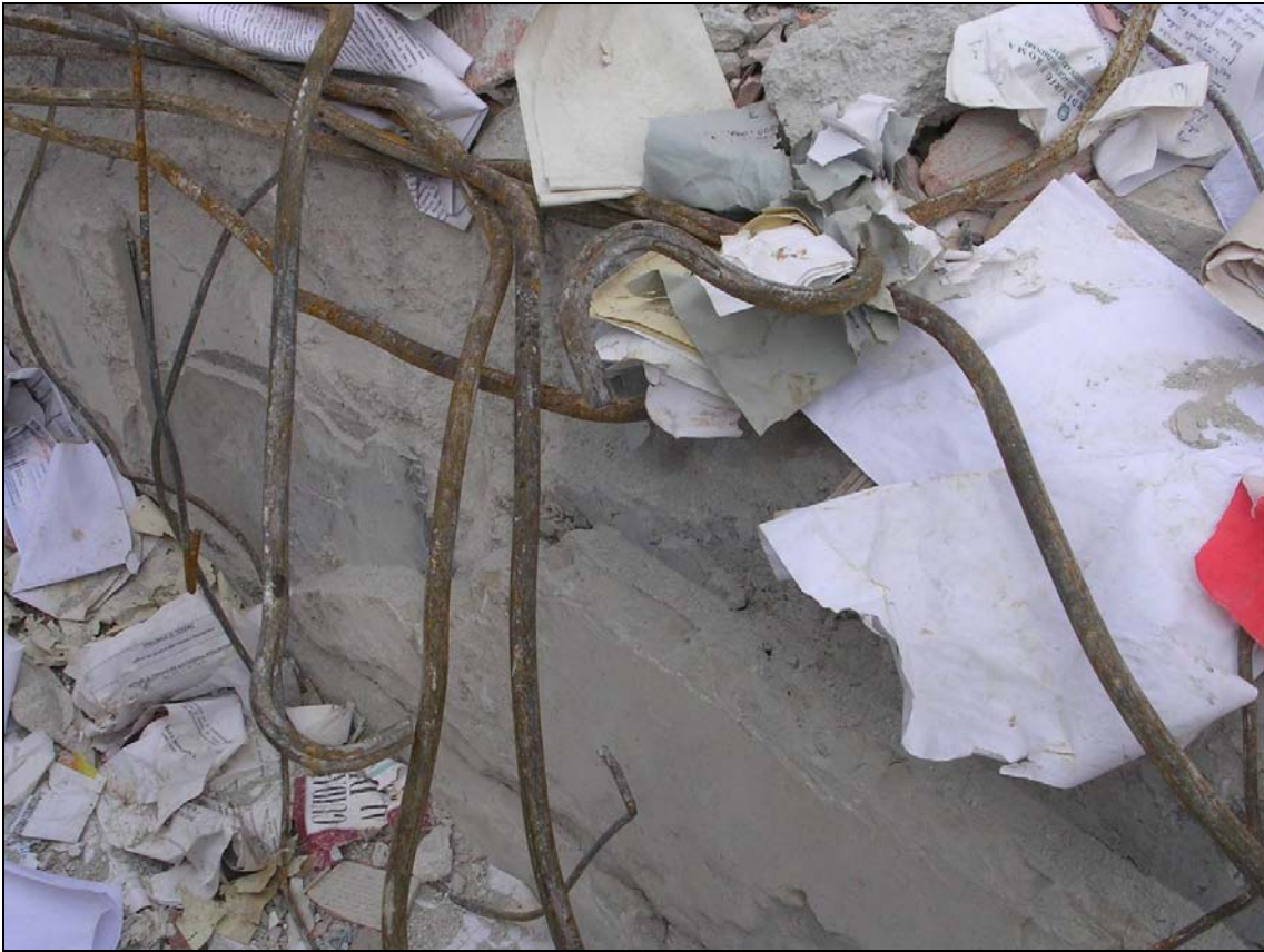
Figure 2. “Smooth iron bars” used before 1980 R.C. building. The use of this technique is not due to an imprudence or incapacity, as media have said, because until 1976 (Friuli earthquake, Mw=6.4) the seismic code didn’t prescribe “improved adherence iron bars”.
