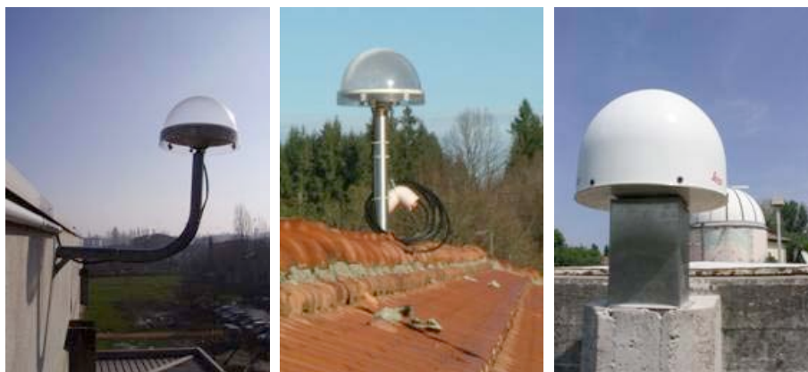
Figure 2 Mo05, Mo02 and SGIP antenna installations.
