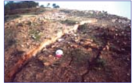
Figure 5: Landslide with cracks in Ait Daoud area
