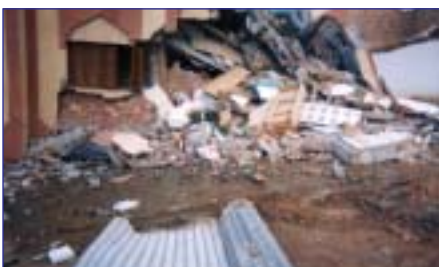
Figure 3: Photos of damage in modern constructions; total and partial collapse of buildings
