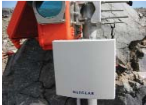
Fig. 6. Directional antenna for wi-fi data transmission to Lipari Island.
