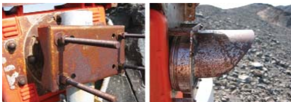
Fig. 10. Gas corrosion effects at Vulcano station.
