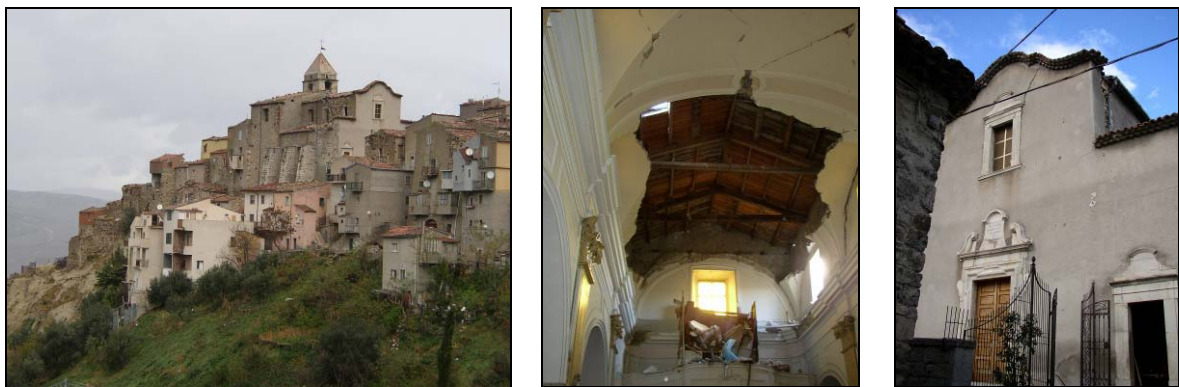
Figure 5: S. Pietro in Vincoli church – Castellino del Biferno (CB): overall view and observed damage
