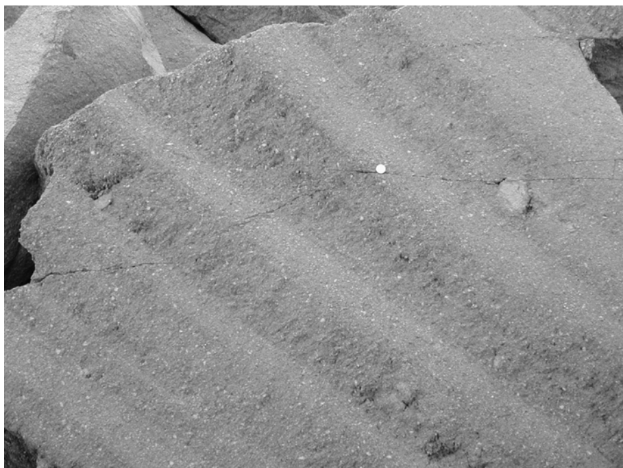
Fig 10: Layers of different porosity in blocks on the dome. Layer thickness is in the cm to dm range. (picture width approx. 1m)
