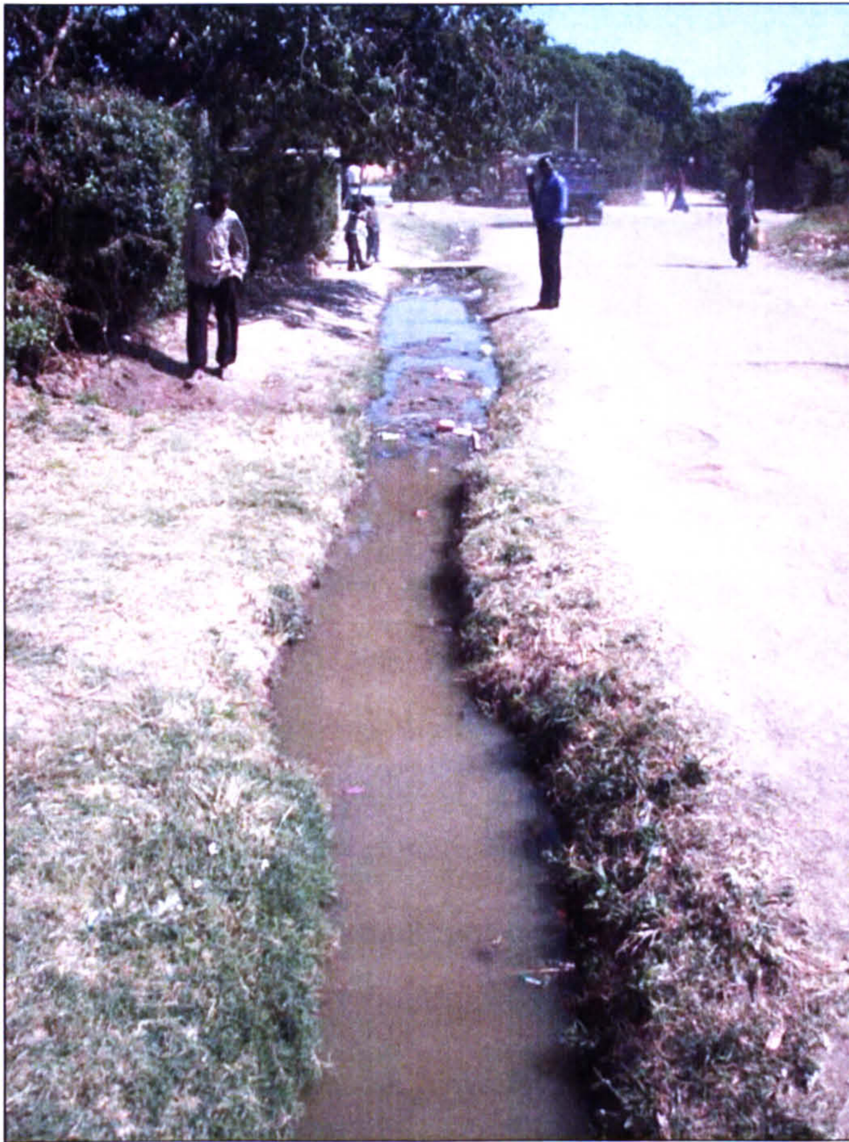
Figure 7.8: Sewage flowing from a blocked sewer in a low cost township in Chingola.
