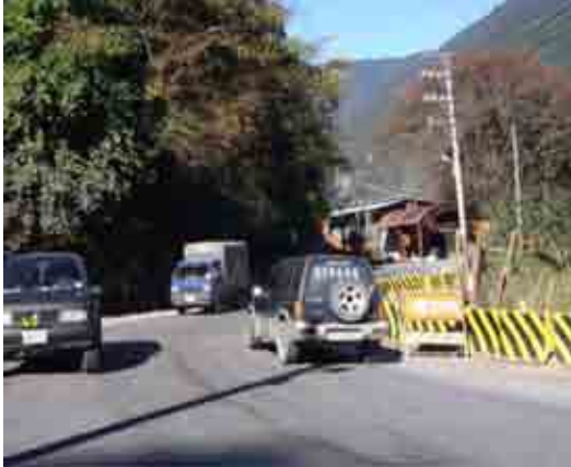
the provincial highways No. 14 in Renai which damage by typhoon in 2008 summer
