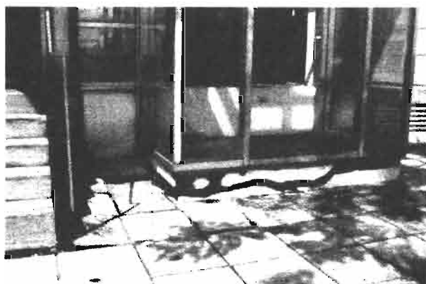
Photo 1 Land subsidence in the suburbs of Bangkok
