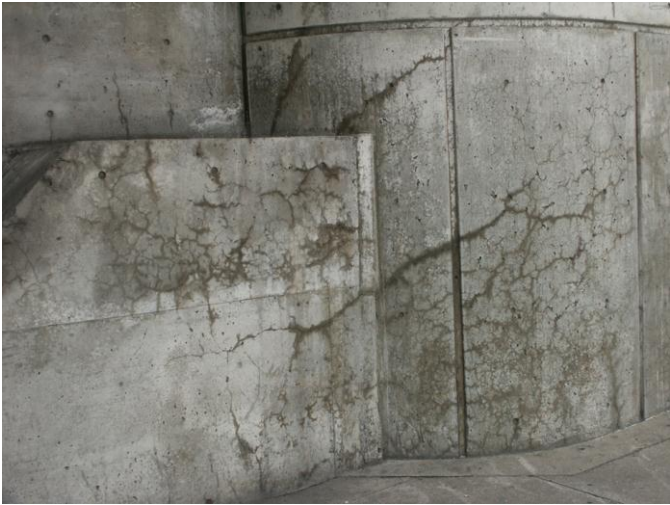
Figure 4: Sidewalk level of large concrete elements showing signs of serious ASR damage.
