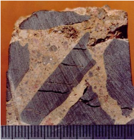
Figure 2: The enemy without – Damage to the near surface zone of concrete on which sodium sulphate was regularly spilt in a production process (the scale at the bottom of the picture is in mm).
