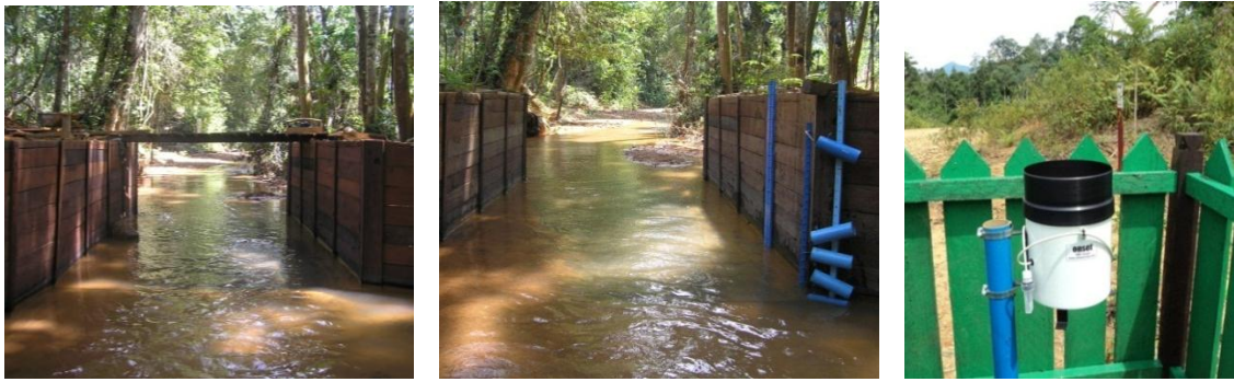
Figure 2.22 Flume weir in the C3 outlet and the rain-gauge.
