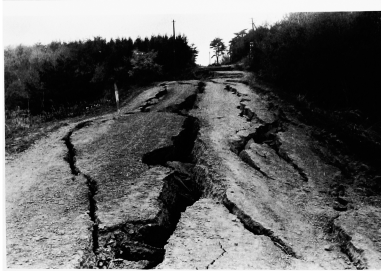
Fig.2 Crack of tensile type in the Tokachioki earthquake, May 16, 1968.
