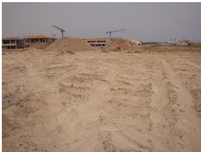
Fig. 15. Compaction of sand due to construction traffic on Algodoeiro.
