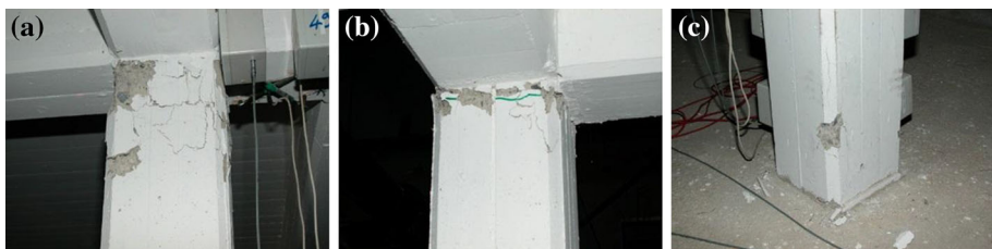
Fig. 4 Visible damage in the specimen after the 0.20 PGA test: a extensive spalling at the top of columns (C3); b light spalling and flexural cracking at the top of corner columns (C1); c base of column C3
