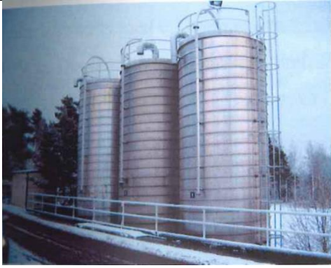
Figure 24 - Storage silos for polyethylene (Hakkarainen, 2007), P. 27
