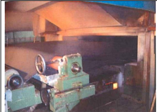
Figure 30 - After the peroxide process, cross-linked polyethylene is coming out of the oven, (Hakkarainen, 2007) P. 29
